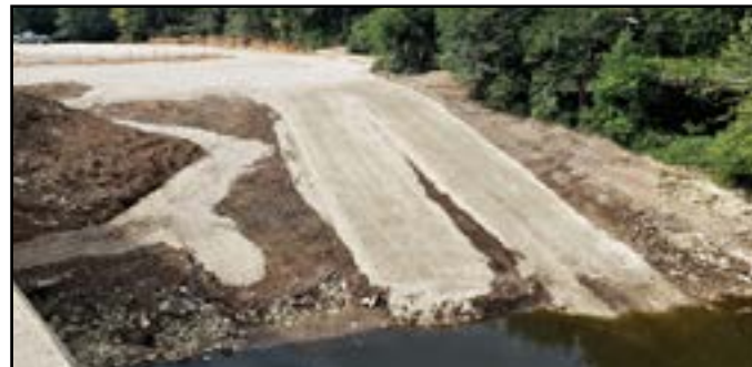
The footprint for upgrades at Iron Bridge Access can be seen now. Work is expected to be completed this spring.
