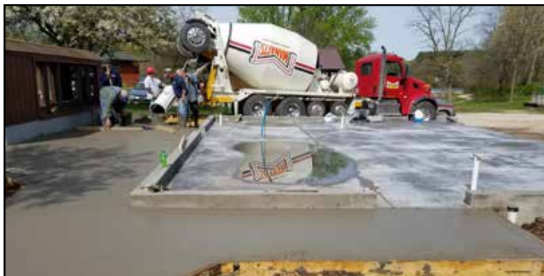
Left: In early May, workers from Klever Concrete pour the floor and sidewalks for the new Wildlife and Animal Care Building at Fontana Park.
